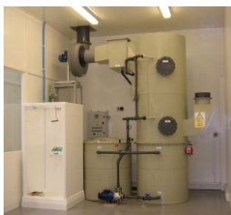
Cabinet with fume scrubbing
